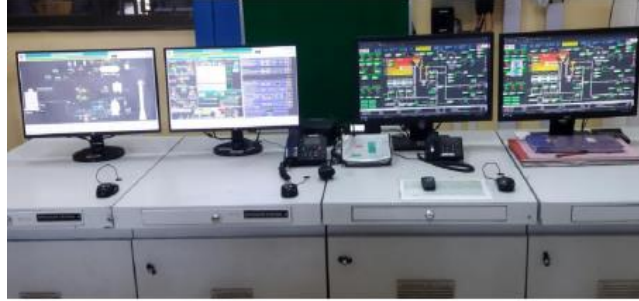
Fig. 1 Boiler control room
