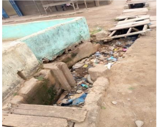
Fig. 15 Clogged and degraded gutters in Seweke
