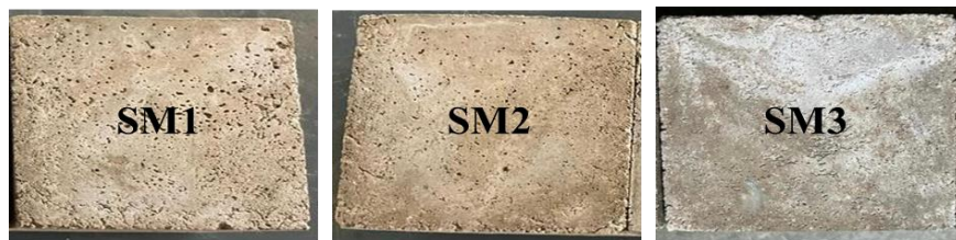
Fig. 7 Visual deterioration of samples SM1, SM2 and SM3 after exposure to sulphate attack for 180 days at 5% sulphate concentration
