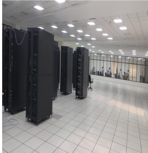
Fig. 5 Data center with LED light fixtures
