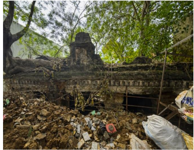
Fig. 9 Dilapidated Heritage Mandapam in Girivalam Path - Thiruvannamalai, Source: authors
