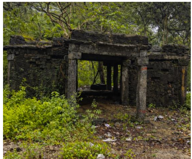
Fig. 8 Dilapidated Heritage Mandapam adjacent to Highway - Gingee, Tamil Nadu. Source: authors
