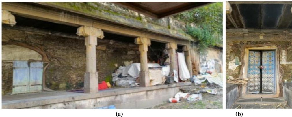
Fig. 25 (a) Dilapidated raised entrance verandah in the front porch of the chatram with vegetation growth in walls, and (b) Entrance of the Gangabhai Chatram, with vegetation overgrowth surrounding the locked doorway.
