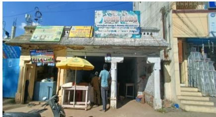
Fig. 14 Heritage Mandapam currently used as a tailor shop and vegetable shop in Kanchipuram, Source: Authors.
