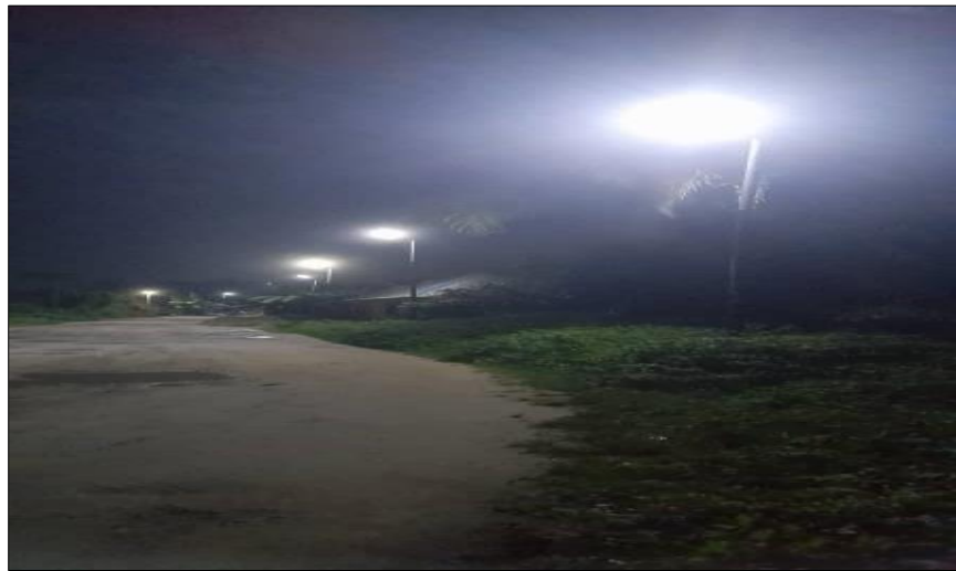
Fig. 1 A photo-view of an installed solar street light in Oleh Town
