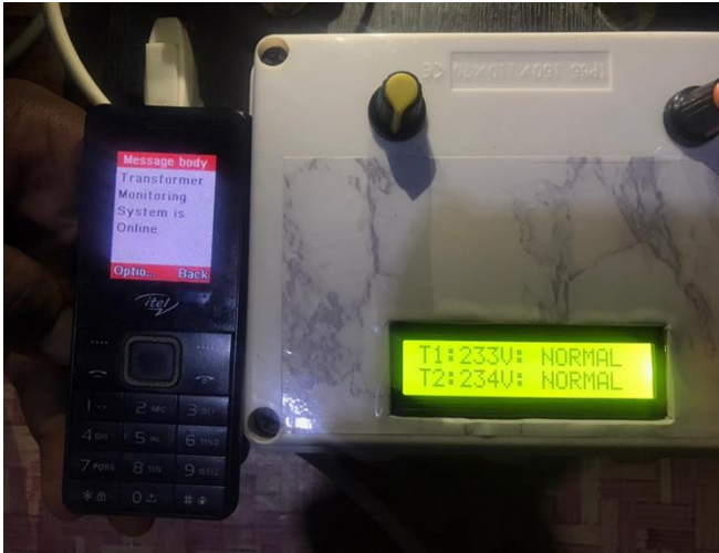
Fig. 13 The picture of the implemented system (transformer 1 and transformer 2) at its normal state
