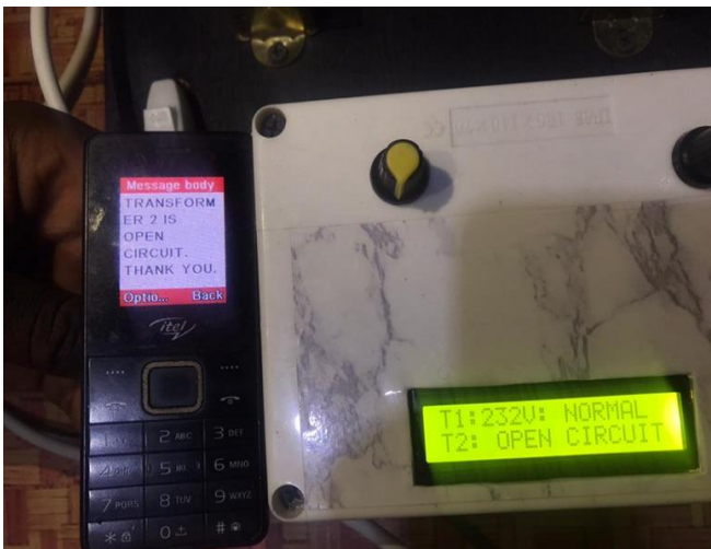
Fig. 15 The picture of the implemented system of transformer 2 in an open circuit state
