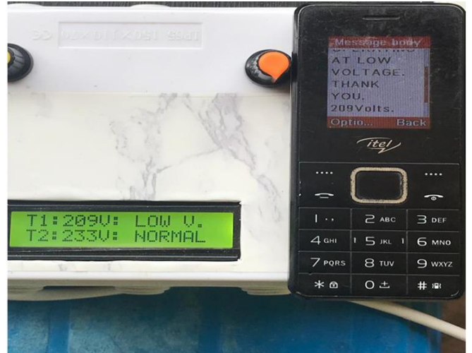
Fig. 16 The picture of the implemented system of transformer 1 at a low voltage state
