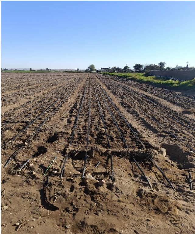
Fig. 3 Piping network for new drip irrigation system
