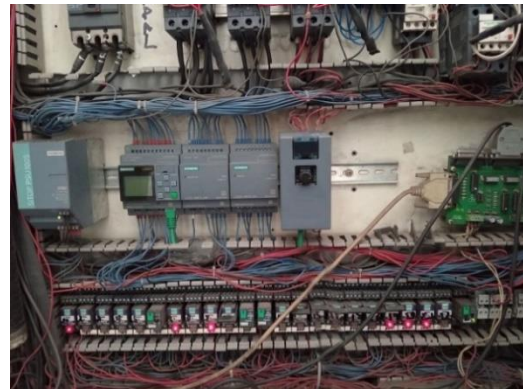
Fig. 12 Control panel with a Logo! PLC and built-in module
