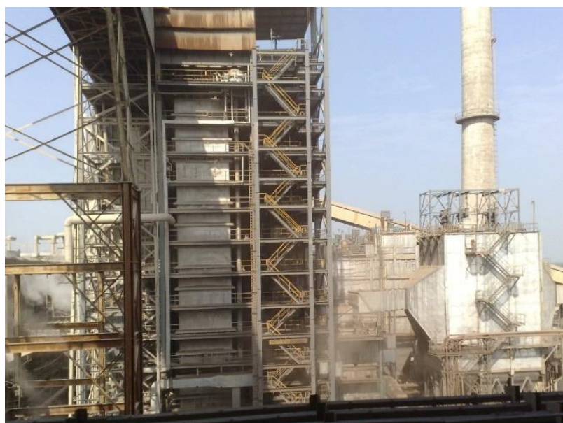
Fig. 4 Boiler system configuration at chemical complex
