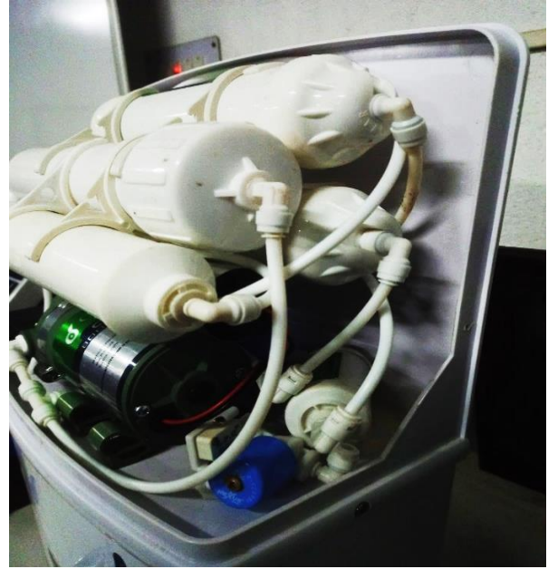
Fig. 7 Water filtration unit (RO booster pump, filters and storage unit)
